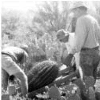
Tierra Madre: Participants take part in the construction of a single-family home using non-traditional building materials. (Las Cruces, NM)
